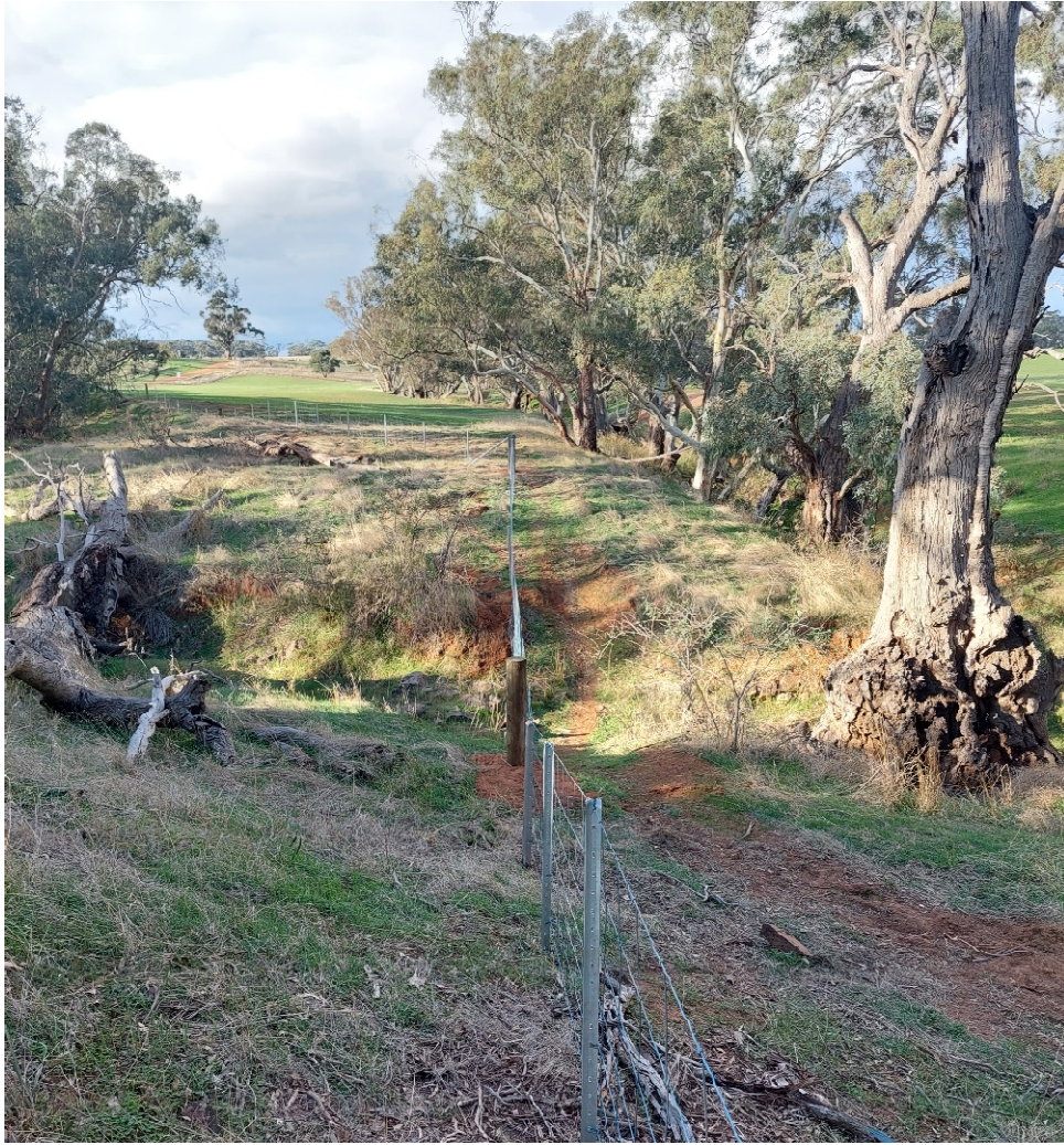
Figure 5: New fencing installed to protect a water reserve in St Kitts while also facilitating public access
