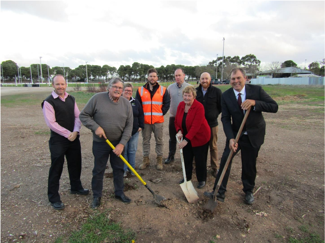
PHOTO CAPTION: The Steering Committee and Project Team Leads for the Freeling Agricultural Multi-Purpose Centre gather on site to mark commencement of the construction phase.
